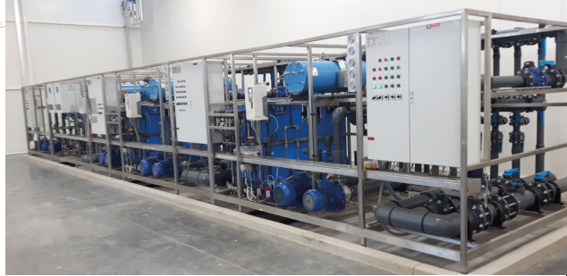
▲ water treatment system
