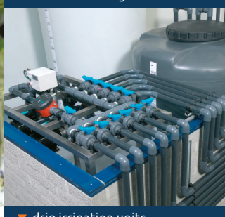
▼ drip irrigation units
