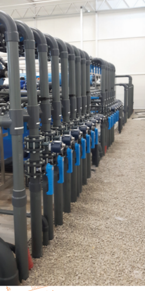
▼ irrigation valve set
